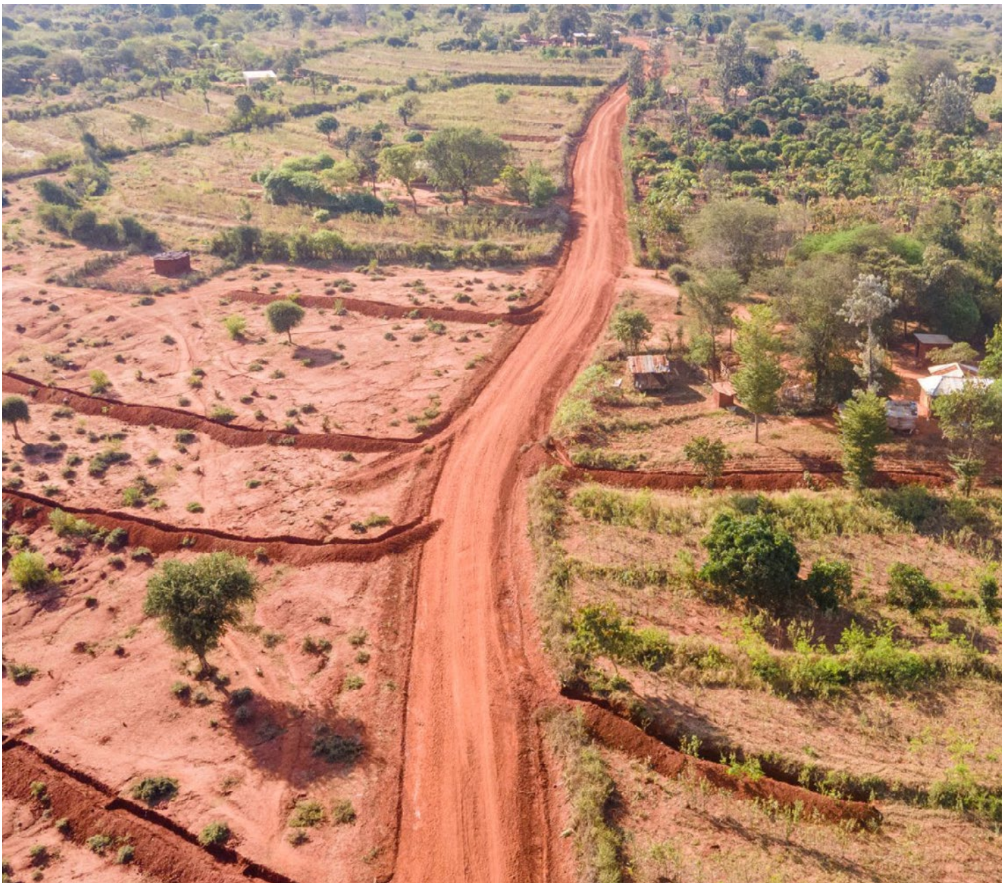
NBS, including run-off harvesting measures, installed along three kilometers of road for the "Drain to Gain Project", Kenya. Photo by MetaMeta.
